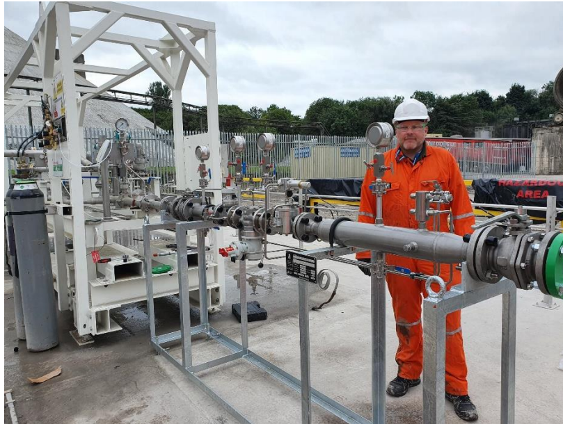
1FTPS Hydrogen Control Skid
